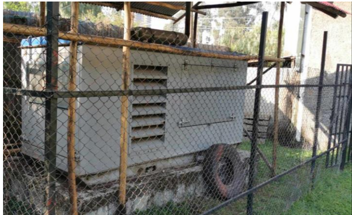
Olaf has done maintenance and repair on the generator.
